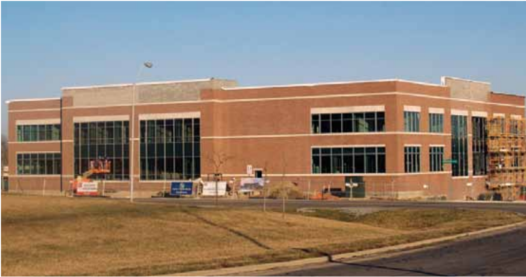
The 66,000-square-foot, three-story building under construction on the northeast side of the Wright State University campus will offer a full array of physician care, including new neurology and sports medicine practices, as well as the existing practices in orthopedics, family medicine, geriatrics, and dermatology.
